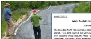
Figure 1: Differential settlement associated with permafrost thaw along an abandoned section of Northwest Territory Highway 4, east of Yellowknife
